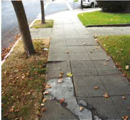
roots raising sidewalk
